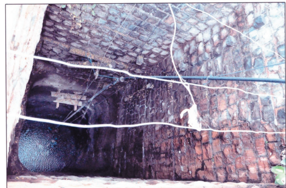
Photograph No 3 – Showing depth of water and narrowness of construction near the base of well.
